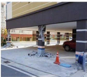
Fig. 1. Failure of Column in Piloti Building
